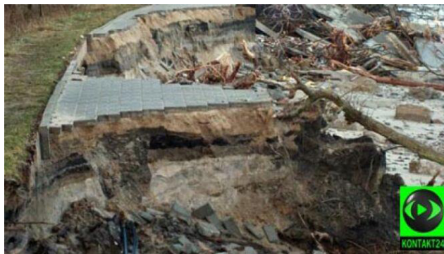
Fig. 5. Destroyed bike path in Kołobrzeg after a storm
